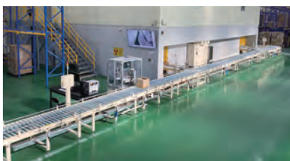
E Plant : E-Beam Irradiation Facility
